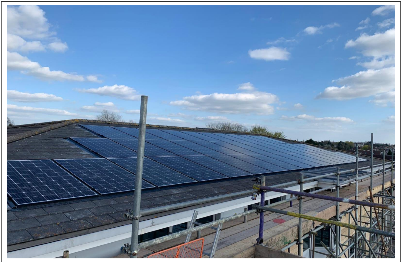
Picture 1. PV installation on Ron Groves House, Kidlington
